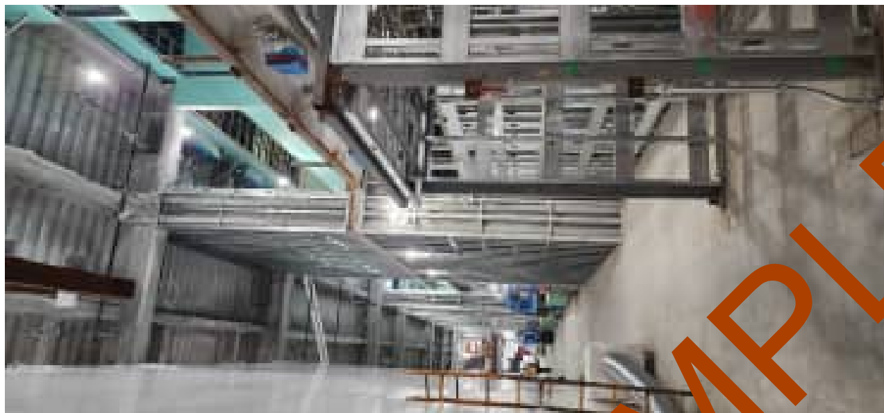
1st level - Interior metal stud framing - spray applied - fire proofing in progress
