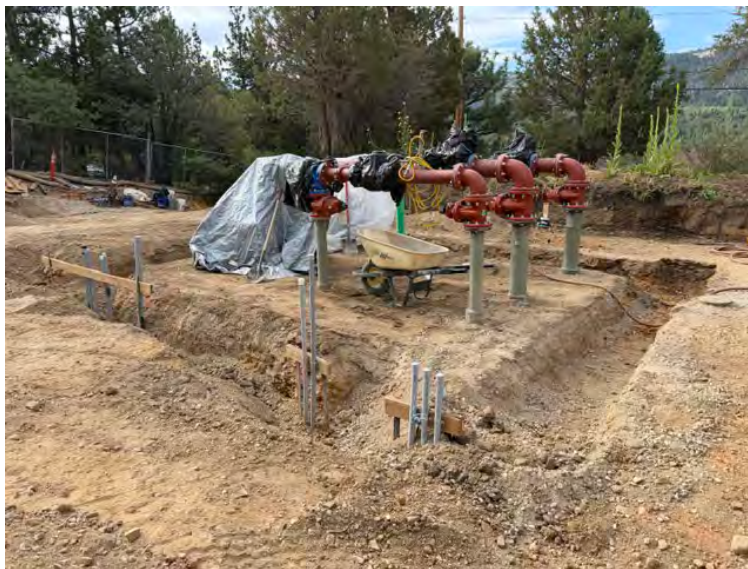
Above ground piping
