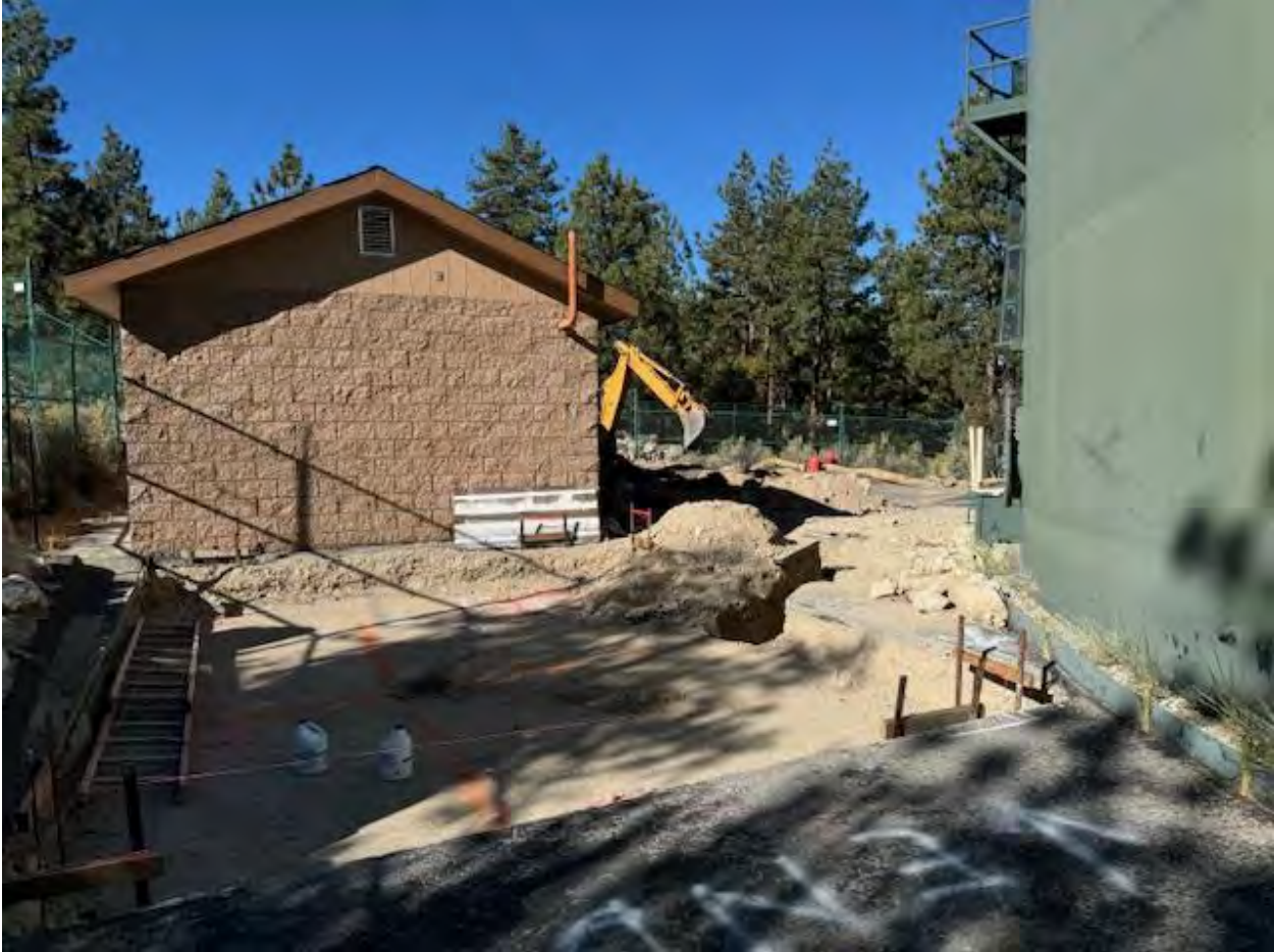
Pontell Hydropneumatic Tank
